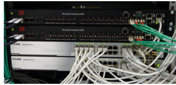
10 Gbit and 1 Gbit switches
