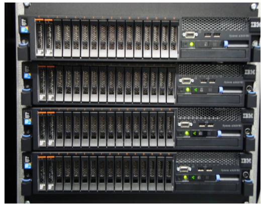
TSM/HSM storage servers
